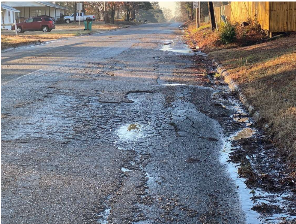
Southbound Lane south of 43 rd Street has severe rutting and failure for a considerable distance.
