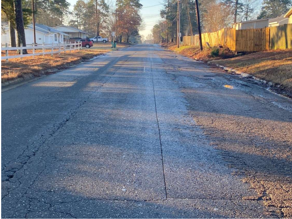
Typical Section of County, Concrete Curb and Asphalt Pavement, patching has been performed numerous times.
