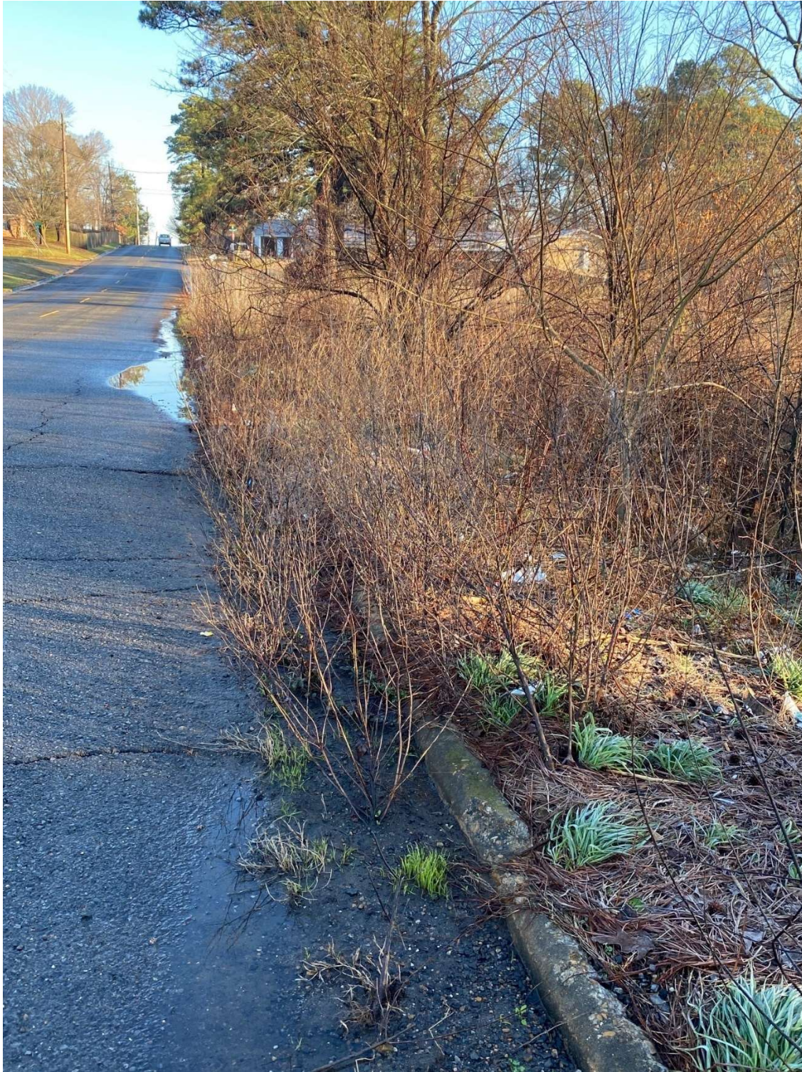
Northbound Lane near the Wal-Mart has vegetation, accumulation of sediment. Asphalt pavement in this area does not show rutting but rather normal cracking for the age of the pavement.
