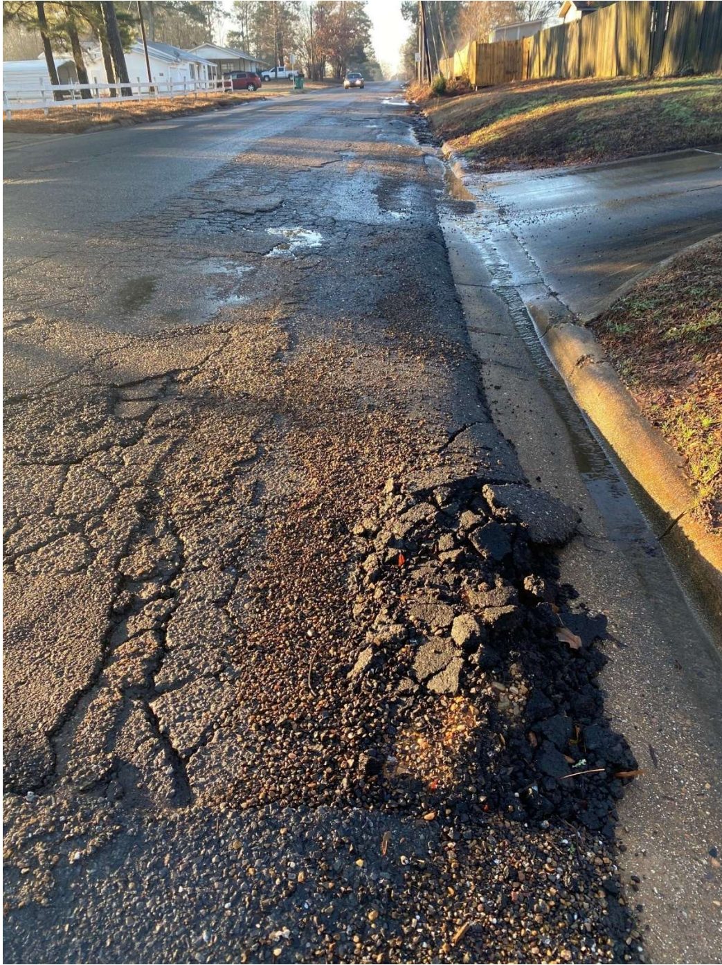
South Bound Lane just south of E 43 rd Street, severe rutting and failure of pavement
